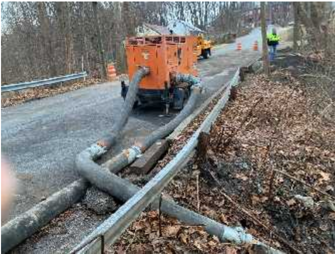
Rented By-Pass Pump
