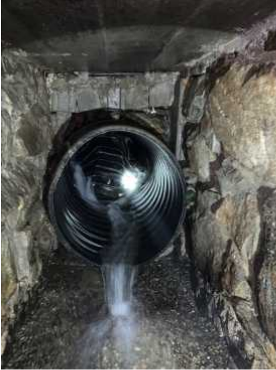
Failed Plastic Culvert Extension (inside of culvert)
